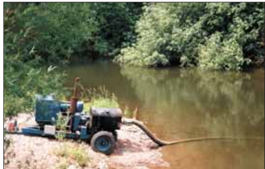
Pump abstracting for spray irrigation at Broadwas on River Teme
